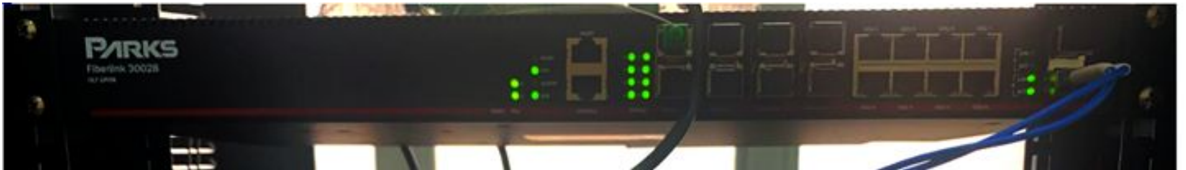
OLT installed on School of Applied Sciences.
